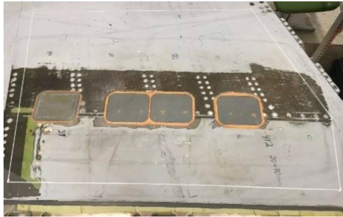
Figure 34 – Bonded repair certification on F-18 wing root (taken from Presentation 13 - Validation and certification of bonded repair on F-18 wing root step lap joint).
